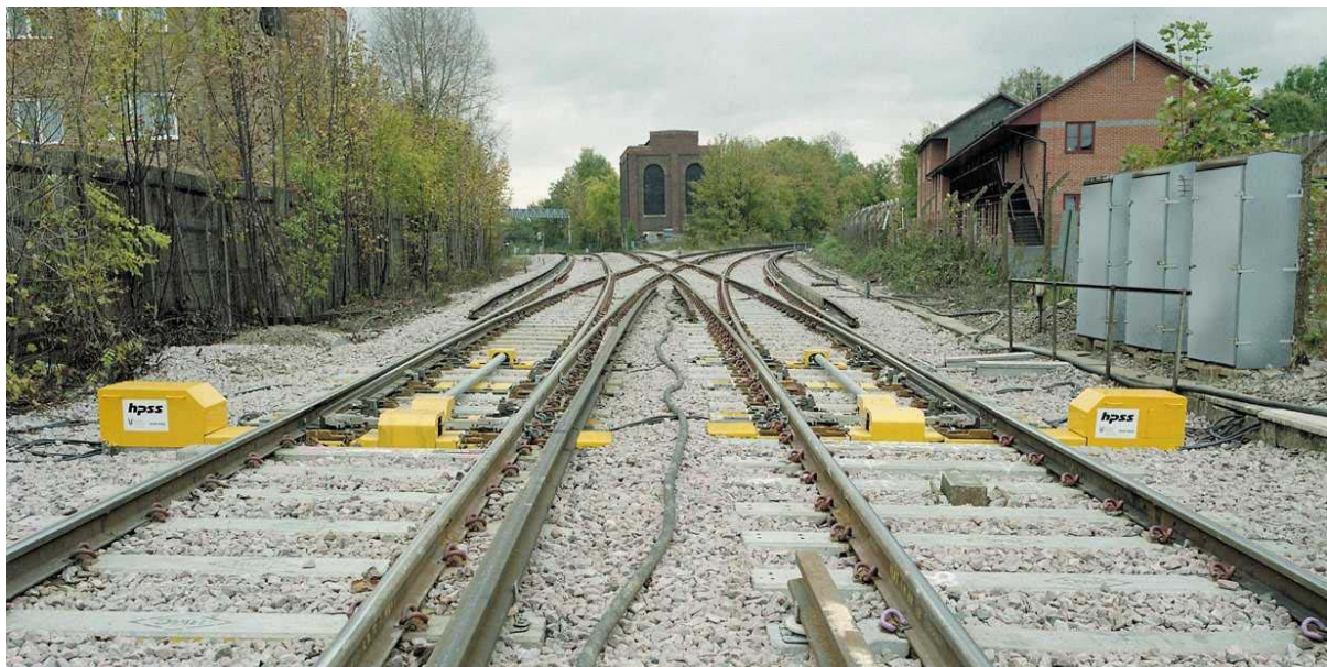
HPSSs Installed At Nunhead Junction (Railtrack Southern Zone)
